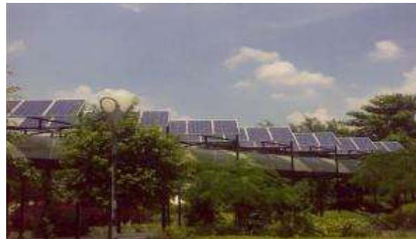
54 kw Solar Power Plant at Bawana
