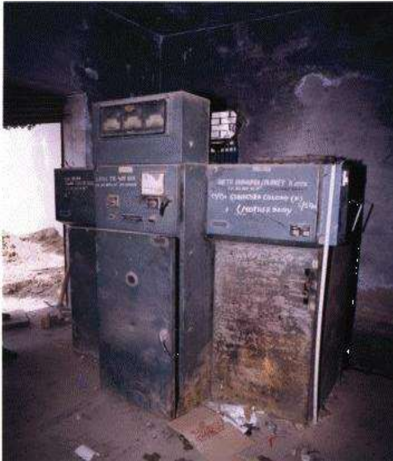
Before : Old Switch Gears
