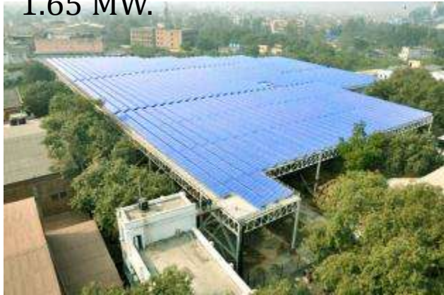
1 MW Solar Project at TPDDL Central Store
