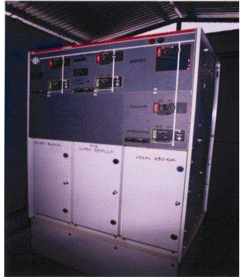
After : New Ring Main Units
