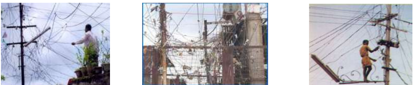
Fig 2: Illegal hooking from the network
